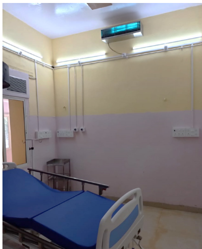
SteraShield - Wall Mounted Upper-Air UVC Device Installed in a Hospital
