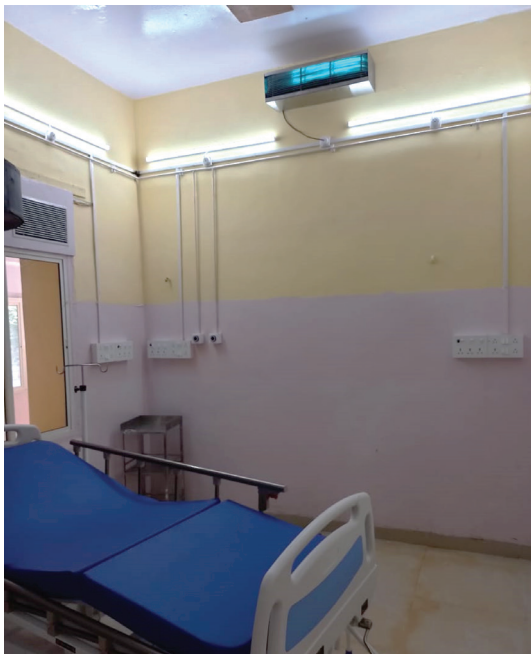
Wall Mounted Upper-Air UVC Device Installed in a Hospital
